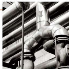
Industrial Piping Systems
