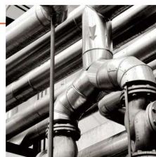
Industrial Piping Systems
