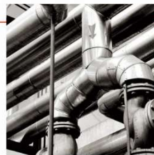
Industrial Piping Systems
